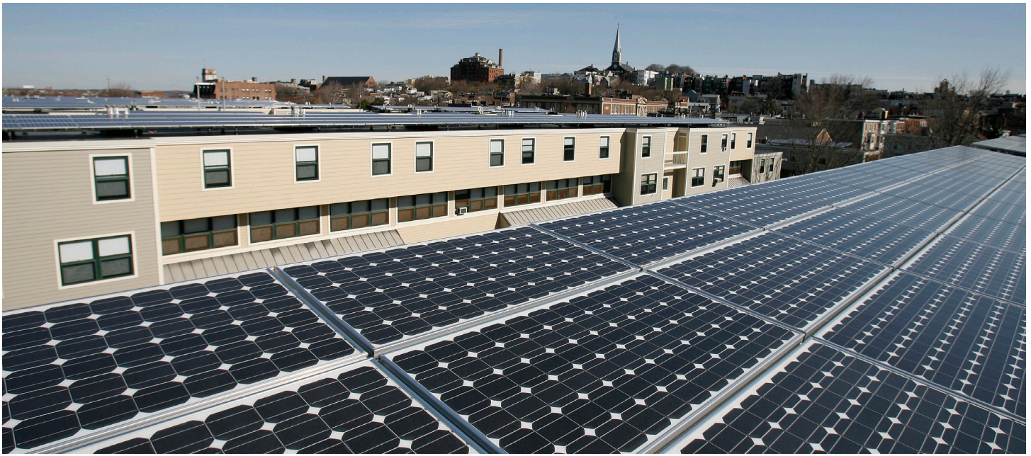
A solar installation on sixteen buildings at Mishaawum Park Apartments in Charlestown, Massachusetts, serves 337 units of affordable housing.
