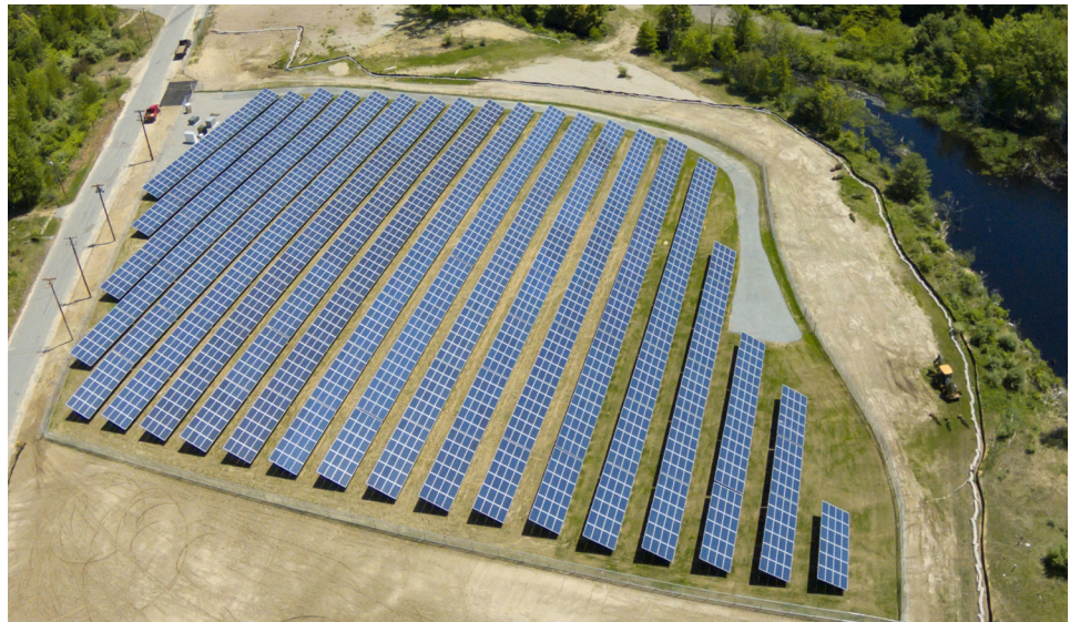
This 986 kW solar farm in Gardner, Massachusetts, serves an affordable housing community, a sheltered workshop, an elderly housing complex, and a local business.
