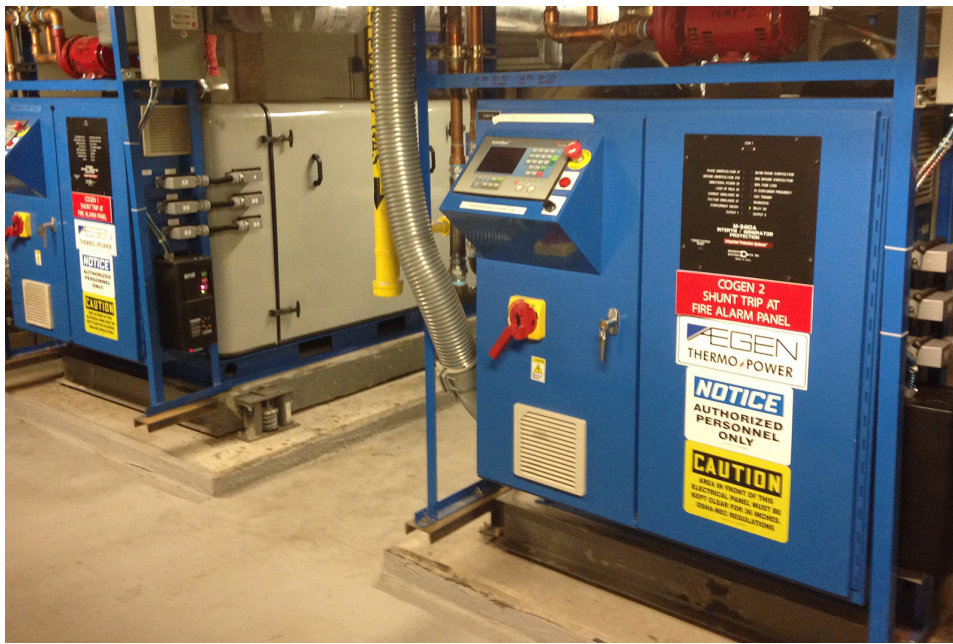
One of two cogeneration units at LB Johnson Apartments in Cambridge, Massachusetts. These units provide heat and domestic hot water while also providing 56% of the electricity used in this high rise elderly housing apartment building.
